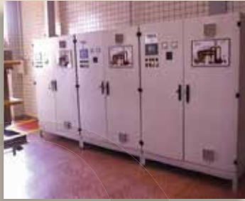
Automatic control panels
